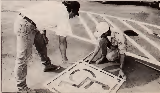
Designated space — Dale Eckley (left) and Tom Shutt, from the Office of Physical Plant, stencil a handicap symbol in a parking space, designating just one of the 107 spots on the University Park Campus that is available for motorists with disabilities. In the near future, 84 more spaces will be created and marked.
